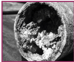
FOG Blockage in Sewer Pipe
